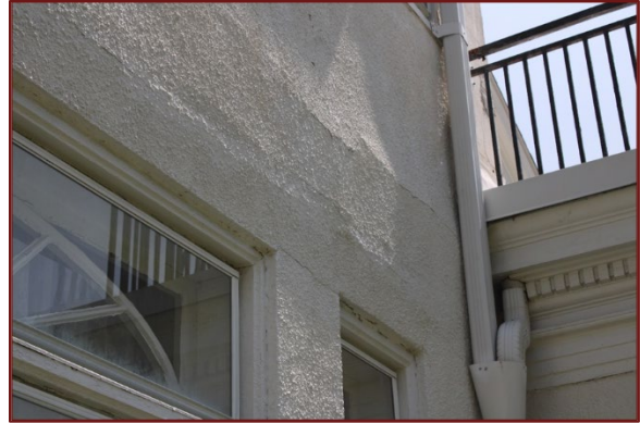
Figure 4-5. Delaminating stucco on the western facade, facing southeast, 2024.
