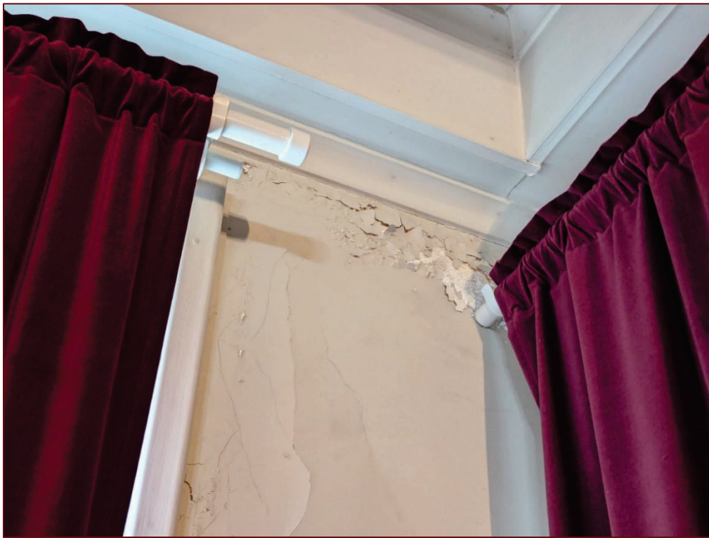
Figure A-19. Example of interior ingress, NW corner of dining room, 2024.
