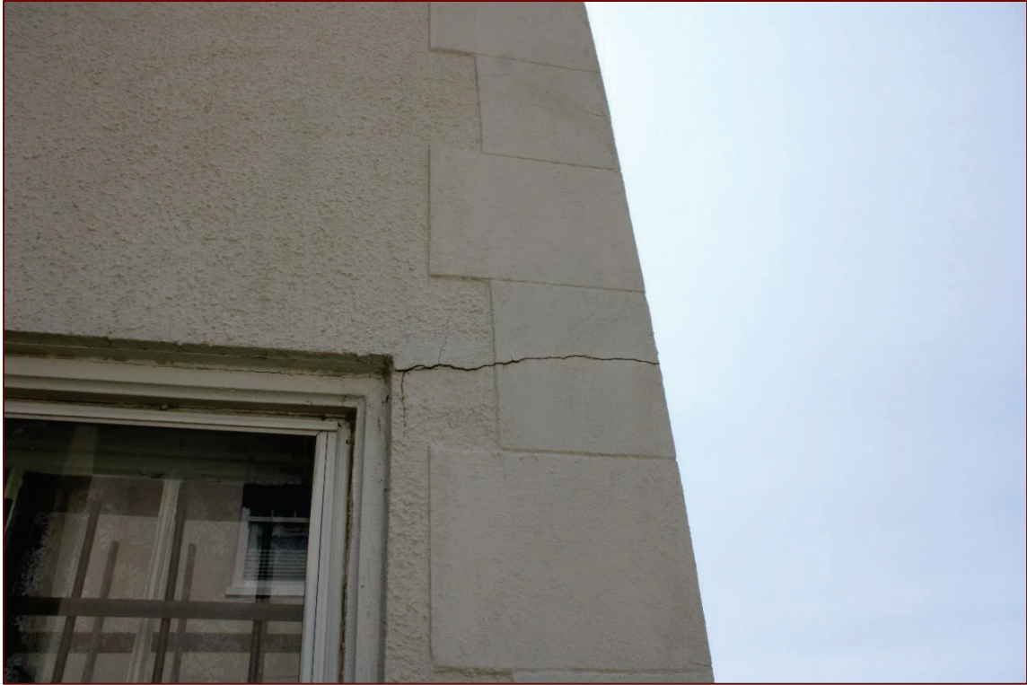
Figure A-5. Example of stucco cracking, western fern facade facing west, 2024.
