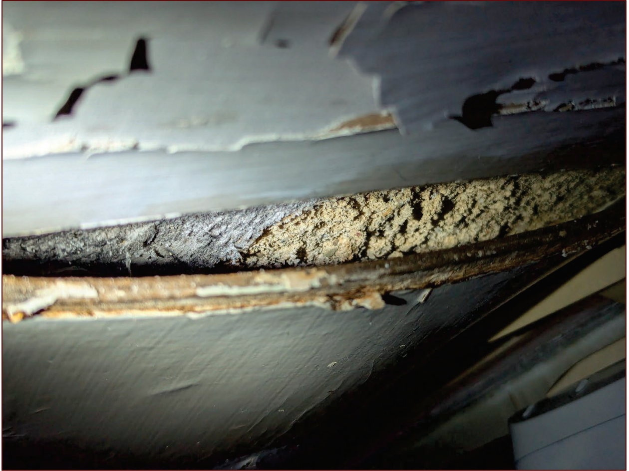
Figure A-24. Example of wall substrate delamination, southwest room, first floor, 2024.
