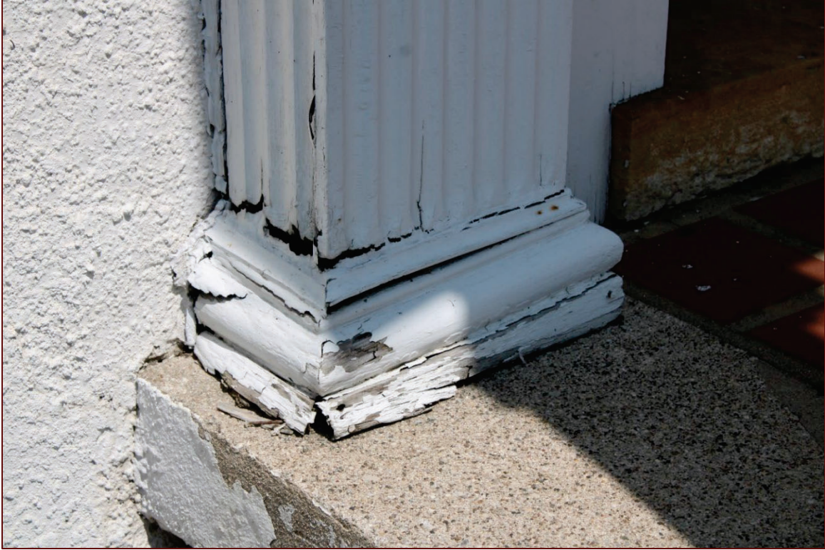
Figure A-14. Example of wood rot, northwestern pilaster, facing north, 2024.
