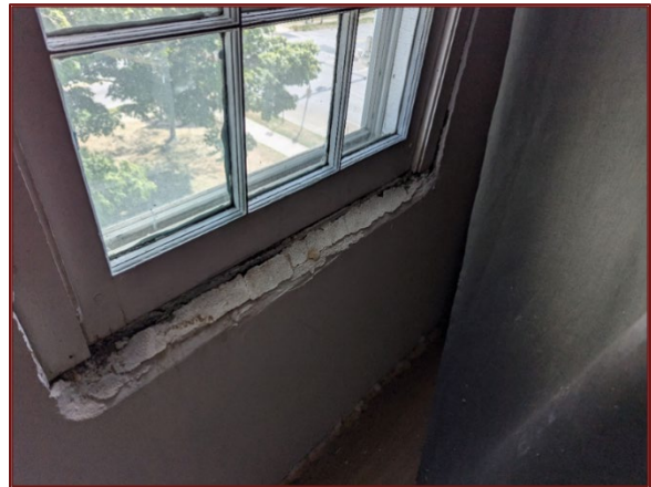
Figure 4-15. Third-floor window showing damage, 2024.
