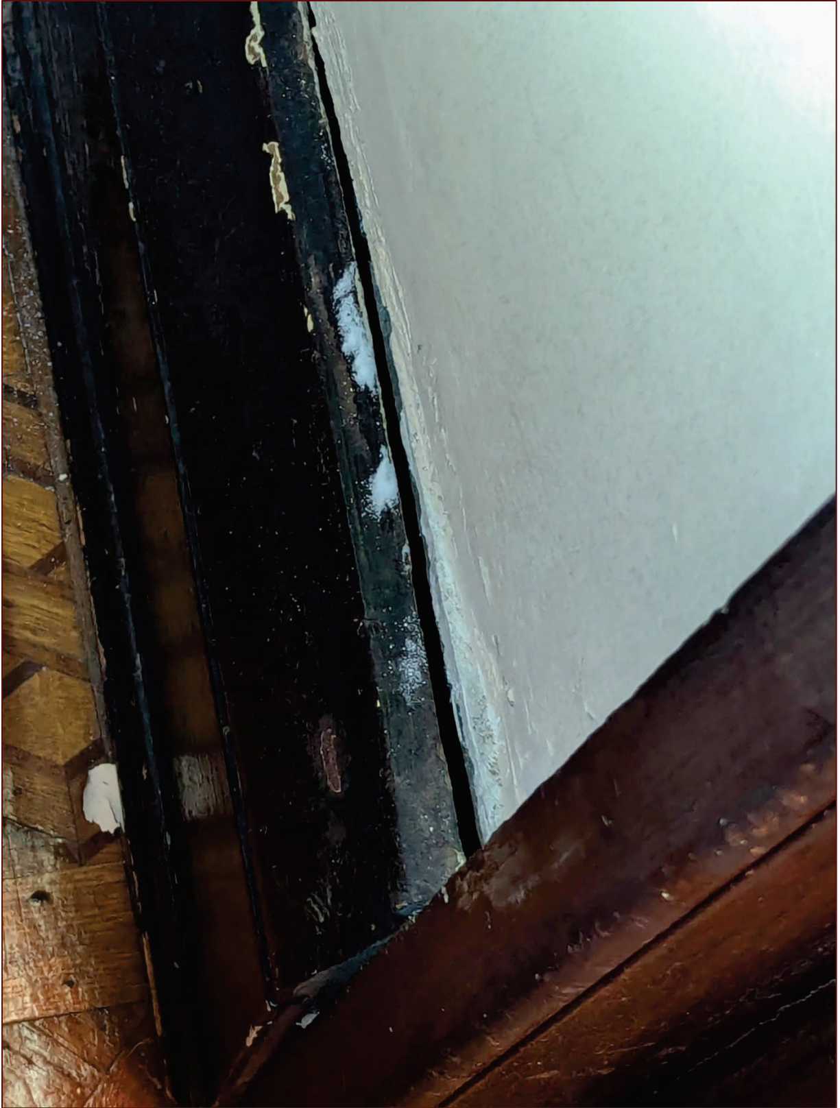
Figure A-23. Example of baseboard/wall separation, southwest corner room, first floor, 2024.
