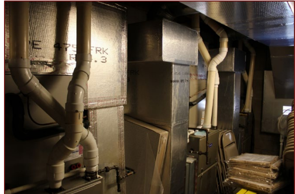
Figure 4-60. Current HVAC units, located in the 2001 built addition, 2025.
