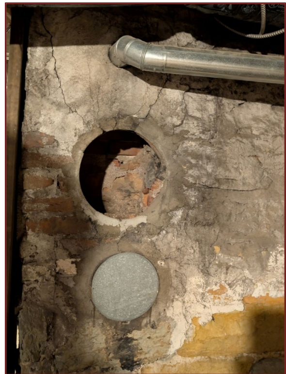
Figure 4-58. Open hole in the basement, requiring attention, 2025.
