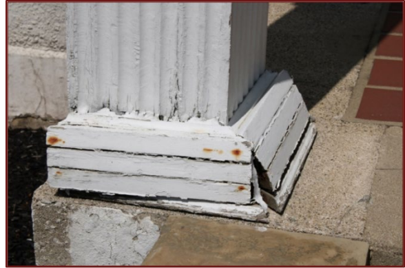
Figure 4-8. Example of wood rot, southwestern entry porch column, facing north, 2024.
