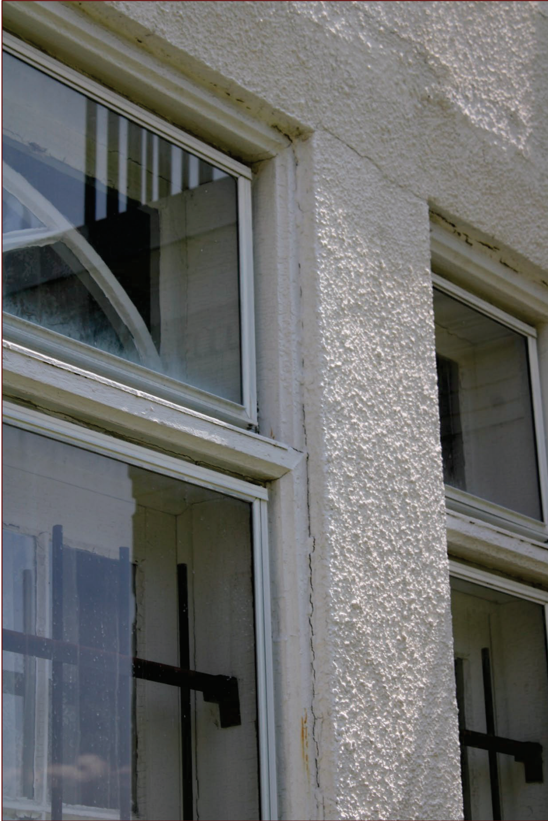
Figure A-4. Example of stucco cracking around window frame, western facade, facing southeast, 2024.
