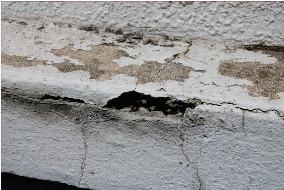
Figure A-6. Example of stucco cracking, western porch, facing east, 2024.
