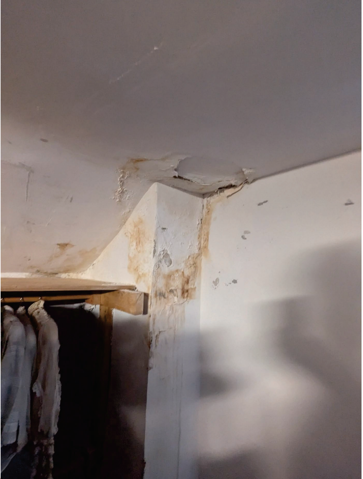
Figure A-21. Example of interior water damage, western room, third floor, 2024.
