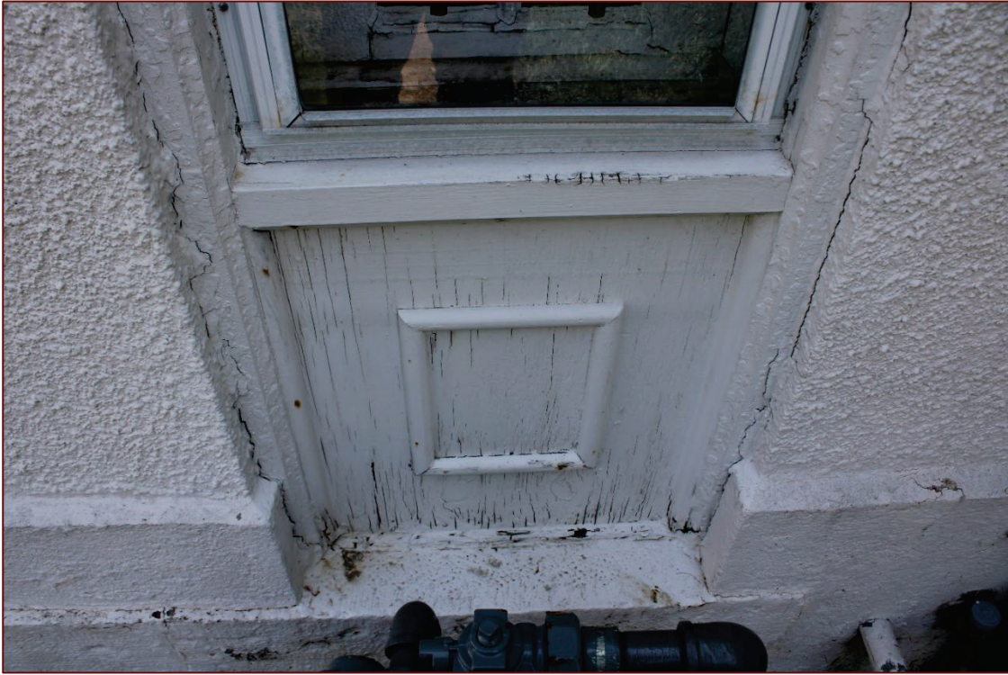
Figure A-16. Example of wood rot and paint failure, western elevation, facing east, 2024.
