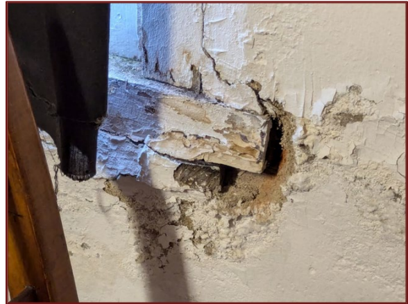
Figure 4-14. Third-floor window showing extreme moisture damage, 2024.
