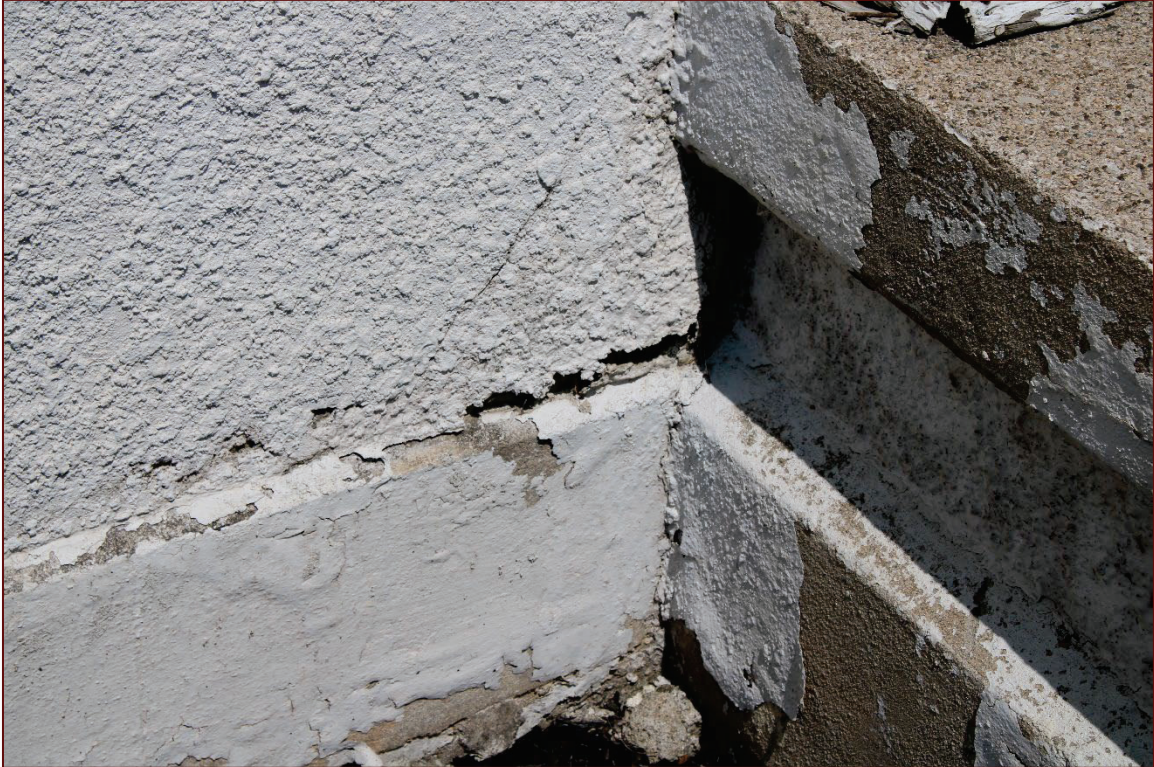
Figure A-10. Example of concrete and stucco cracking, front entry porch, facing northeast, 2024.
