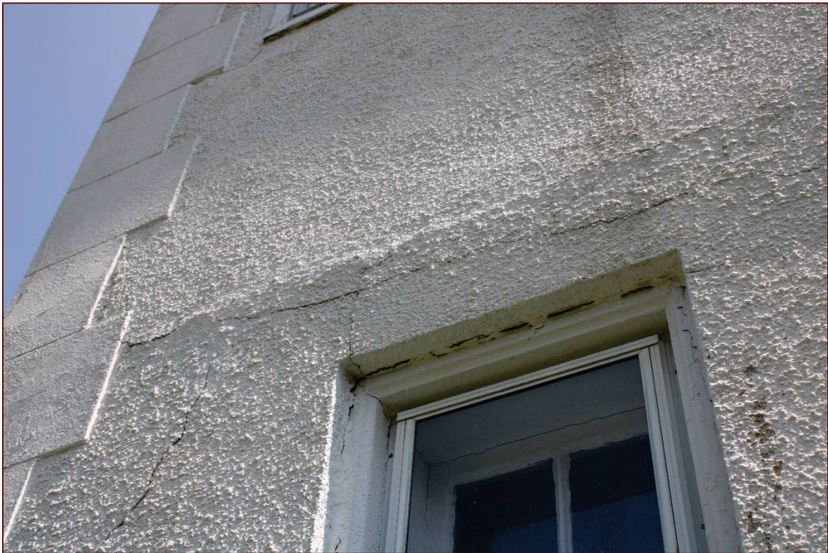
Figure A-2. Example of stucco delamination, west facade, facing east, 2024.
