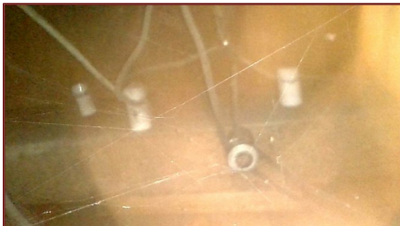
Figure 4-59. Extant knob and tube wiring in the basement crawlspace, 2025.
