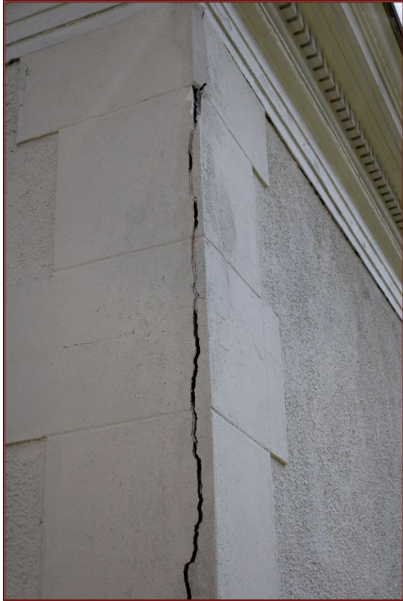
Figure 4-6. Example of stucco cracking, western enclosed patio, facing northeast, 2024.
