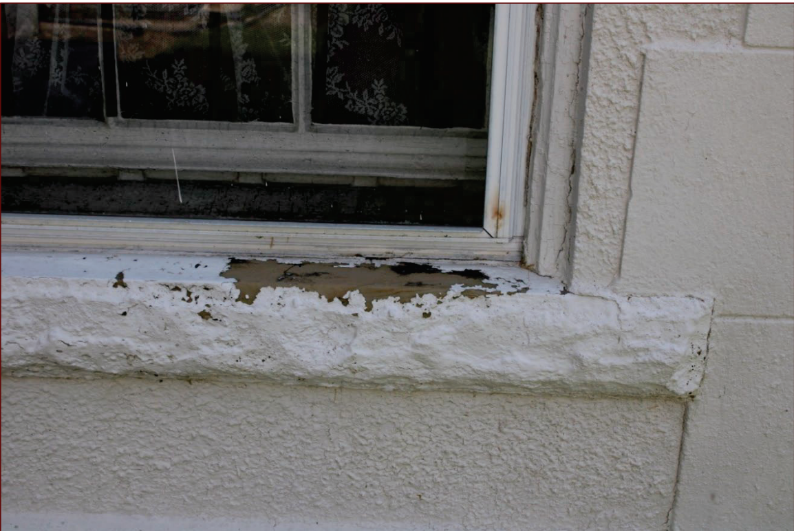
Figure A-11. Example of paint failure on original sandstone sill, western elevation, facing east, 2024.
