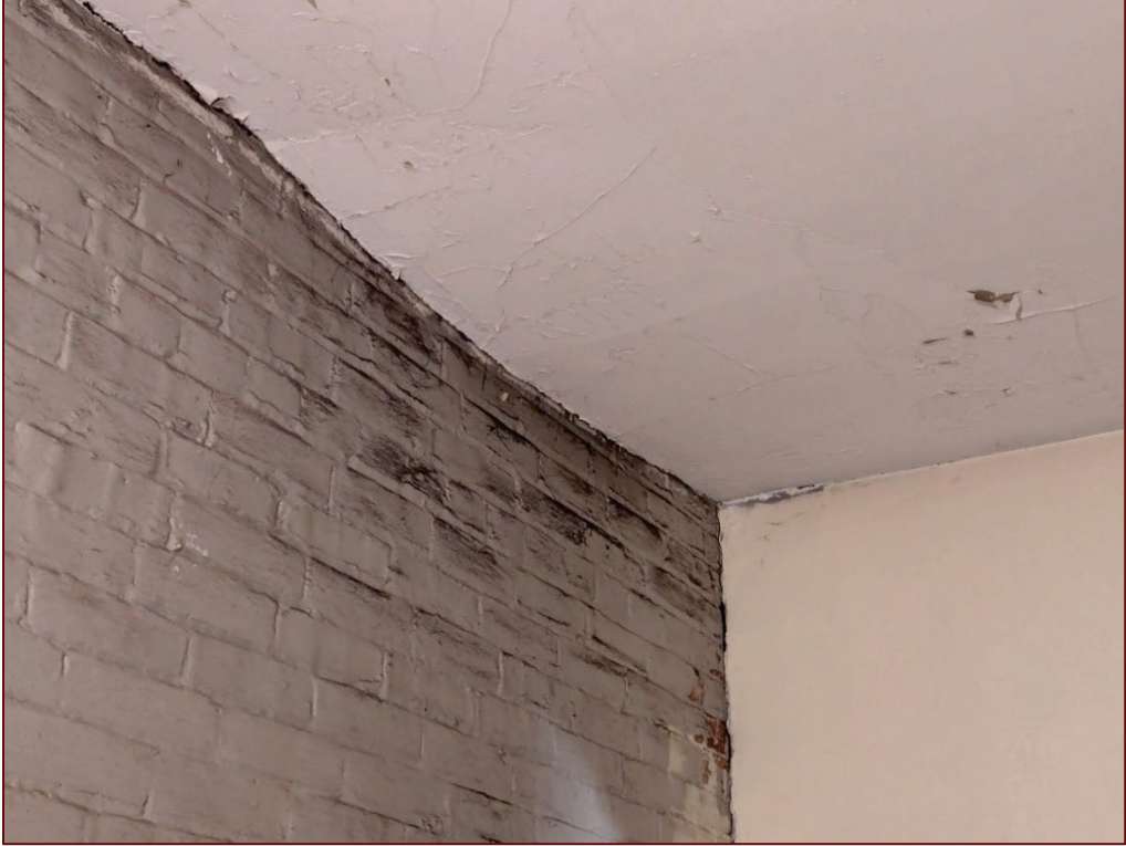
Figure A-20. Example of water damage, Room 19, 2024.
