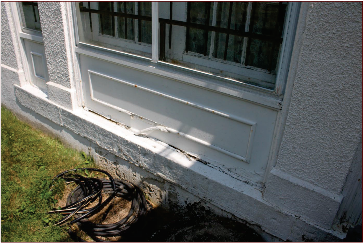
Figure A-15. Example of wood rot and paint failure, western elevation, facing northeast, 2024.
