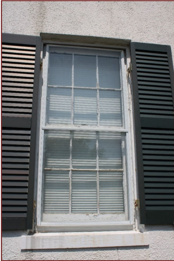
Figure 4-13. Historic, six-over-six window on the western façade, first floor, showing damage typical to most windows in the building, damaged glazing putty, and paint damage, facing east, 2024.
