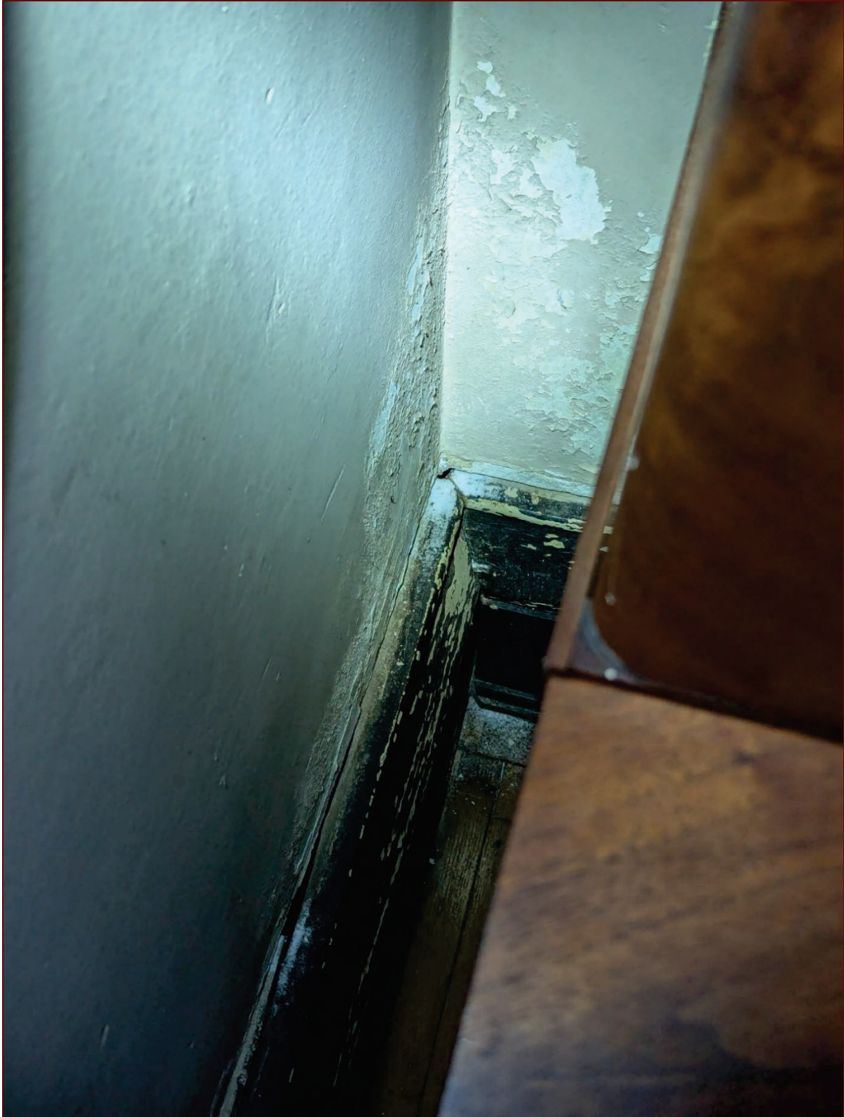
Figure A-25. Example of paint/plaster delamination and cracking, possible humidity issue, 2024.
