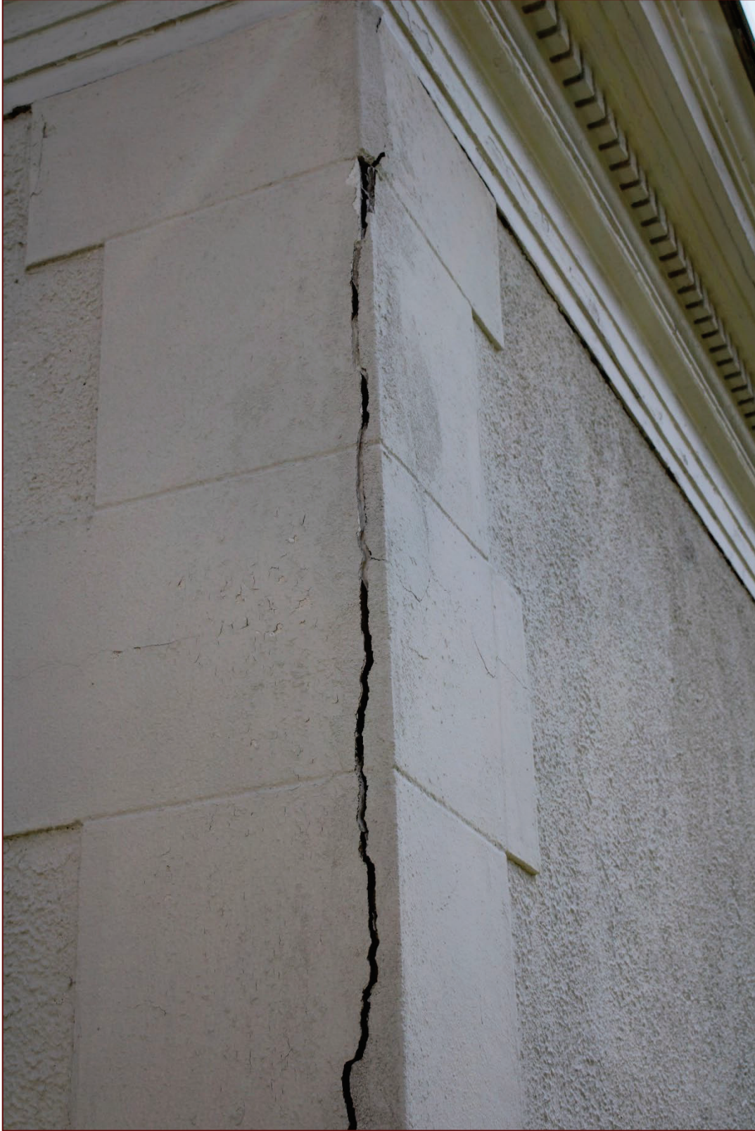
Figure A-3. Example of stucco cracking, western enclosed patio, facing northeast, 2024.
