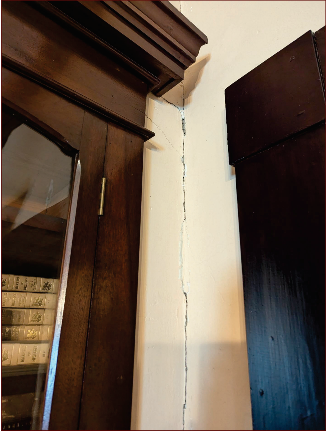
Figure A-22. Example of interior plaster cracking, southwest corner room, first floor, 2024.
