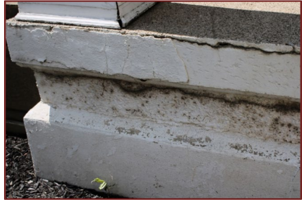
Figure 4-7. Example of concrete cracking, front entry porch, facing west, 2024.
