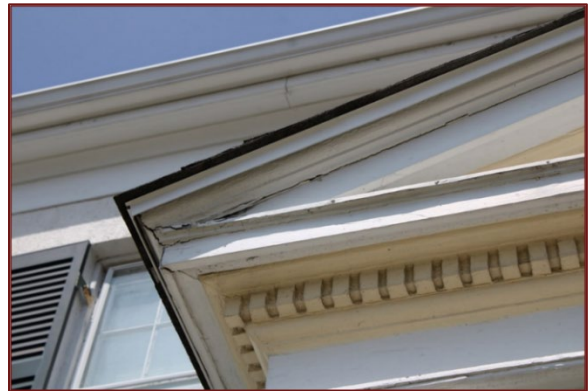
Figure 4-9. Example of wood rot, front entry portico, facing north, 2024.
