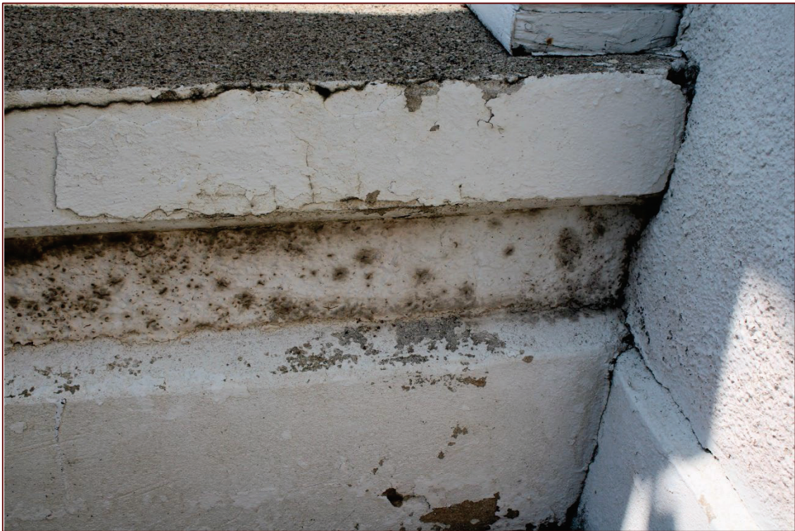
Figure A-9. Example of concrete cracking, front entry porch, facing west, 2024.
