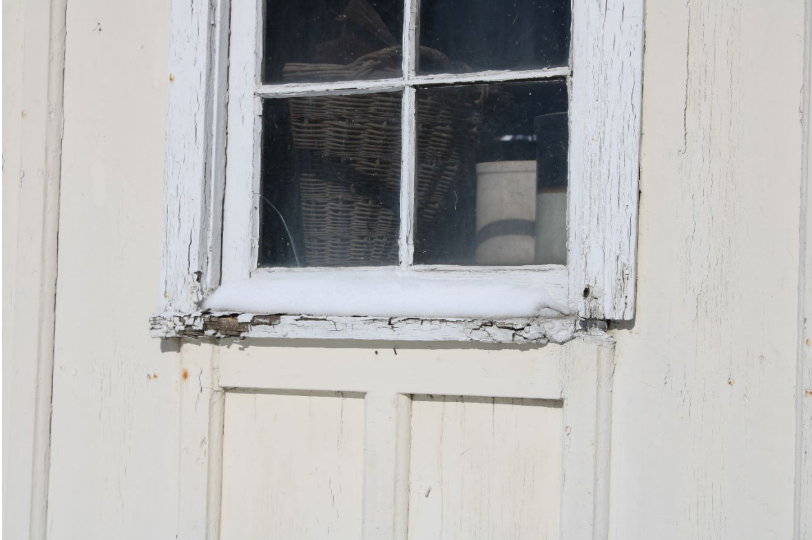
Figure 4-5 Photo of moisture related damage, first floor window, central bay, main façade, facing NW, 2025
