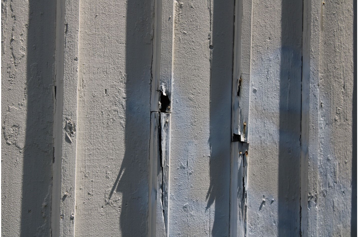
Figure 4-6 Example of wood siding rot and paint failure, western façade.
