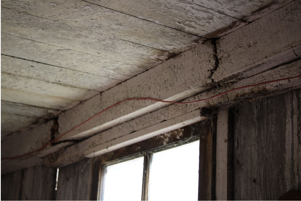
Figure 4-21. Overview of cracked support beam, 2025
