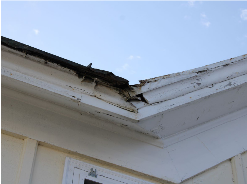
Figure 4-2. Example of the water damage seen on the terne metal roof, facing NE 2024.
