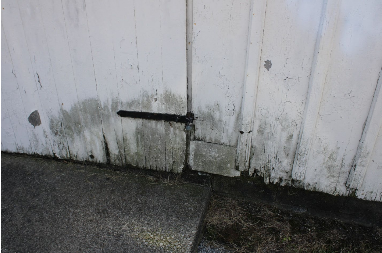
Figure 4-4. Photo showing extensive wood rot on the double doors at the north façade, 2025
