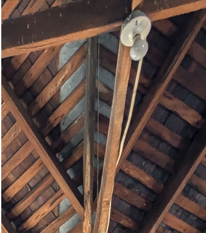
Figure 4-23. Exposed electrical wiring, second floor, 2025
