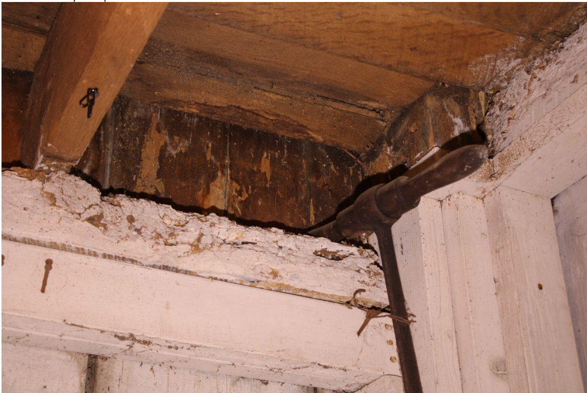
Figure 4-20. Overview of moisture damage on the eastern wall, 2025
