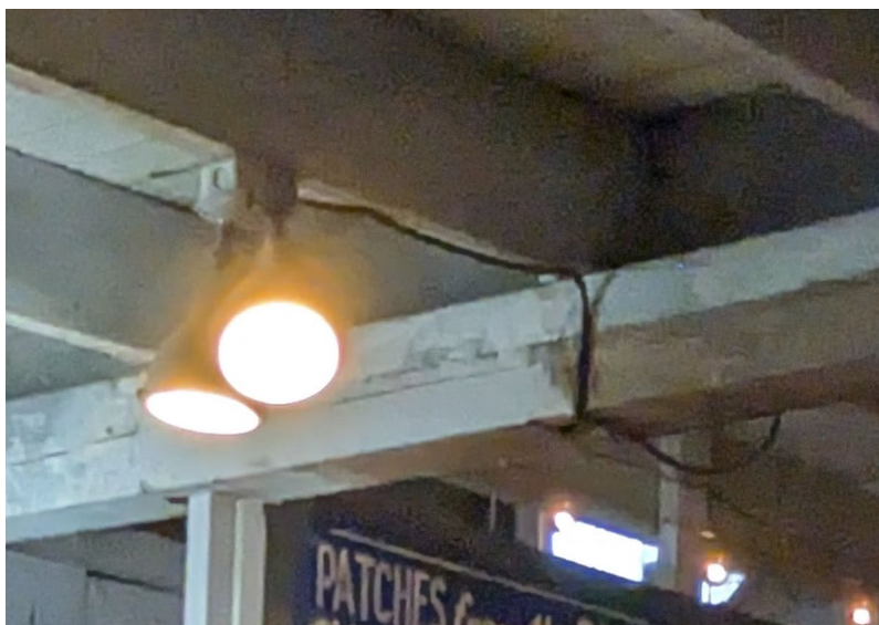
Figure 4-22. Exposed electrical wiring, first floor southern side, 2025
