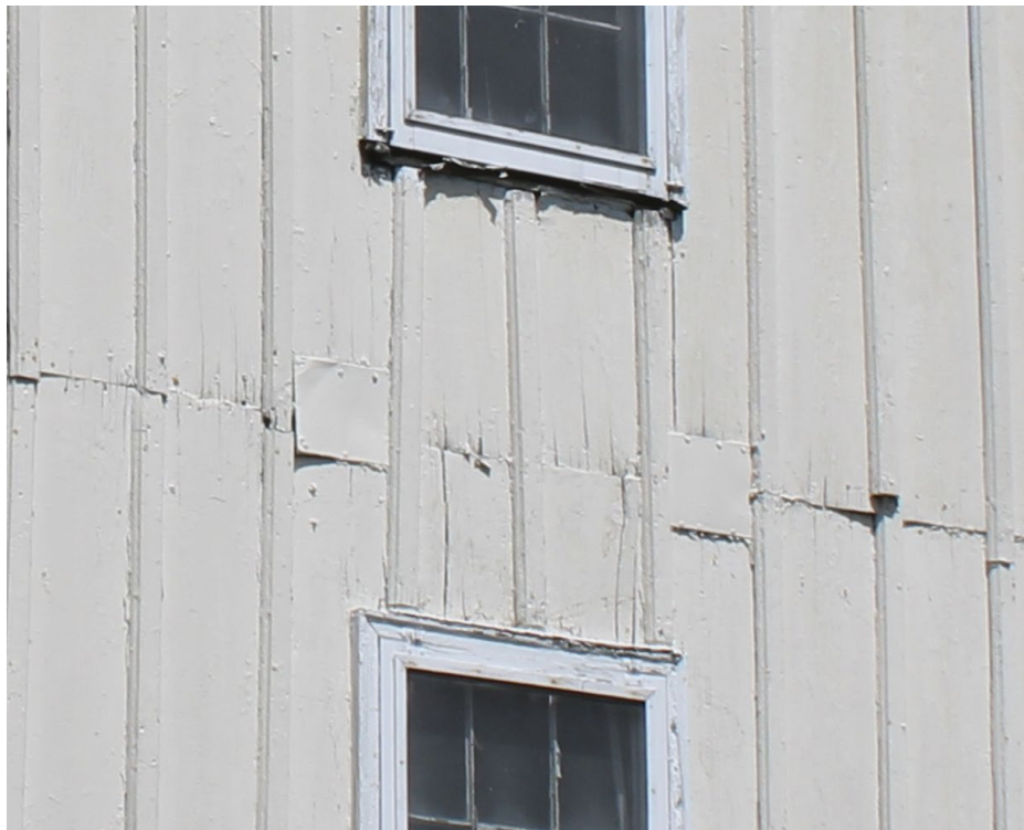
Figure 4-7 Inappropriate siding patches, south facade, 2025
