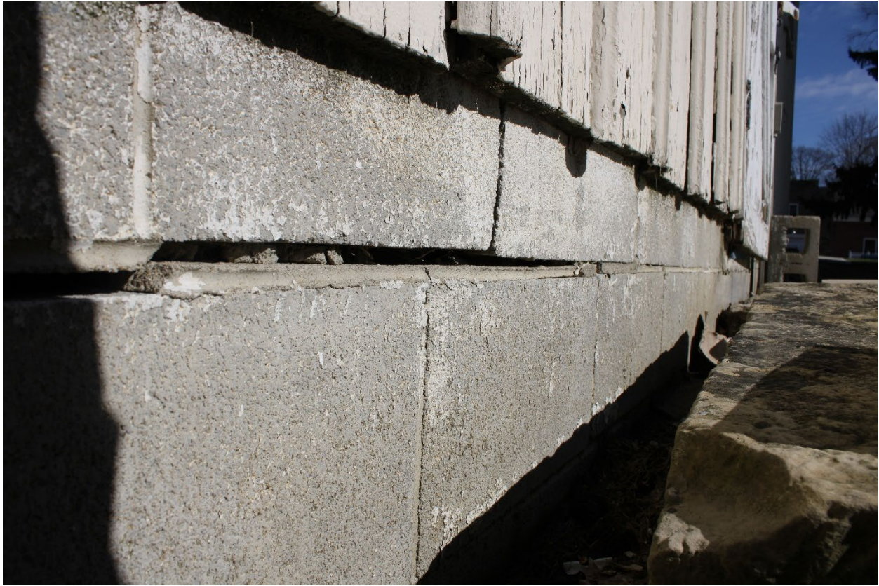
Figure 4-3. Overview of bowing/bulging foundation blocks. 2025
